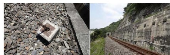
(c) 錨頭掉落
